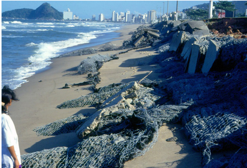
Figure 23. Gabions sea-wall and groins damaged after a storm in 1994 in the northern sector of the Matinhos-Caiobá beach-arc. (see location in Figure 1).
