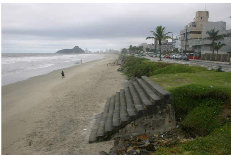
Figure 25. Coastal erosion problem in the northern sector of the Matinhos-Caiobá beach-arc in 2016 (see location in Figure 1).
